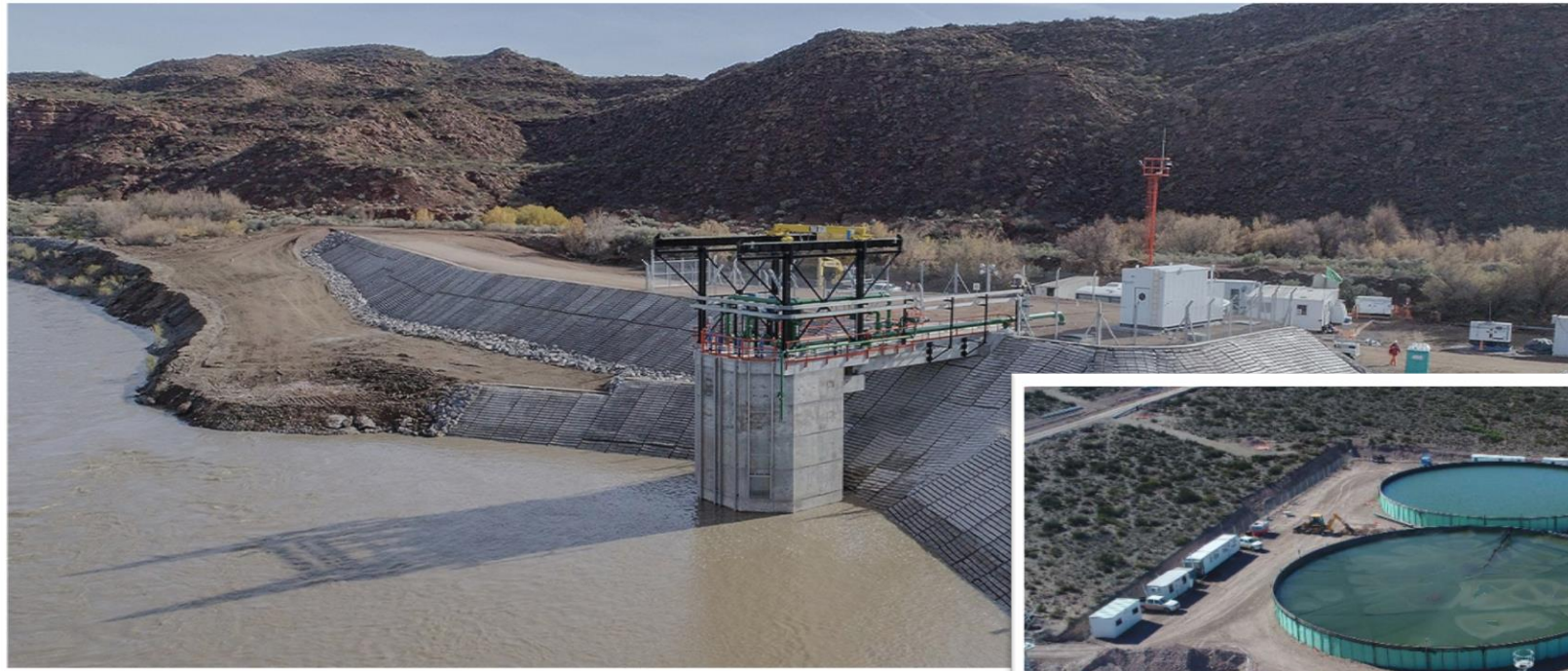
Water Extraction Facility from Neuquén River Filtering station
